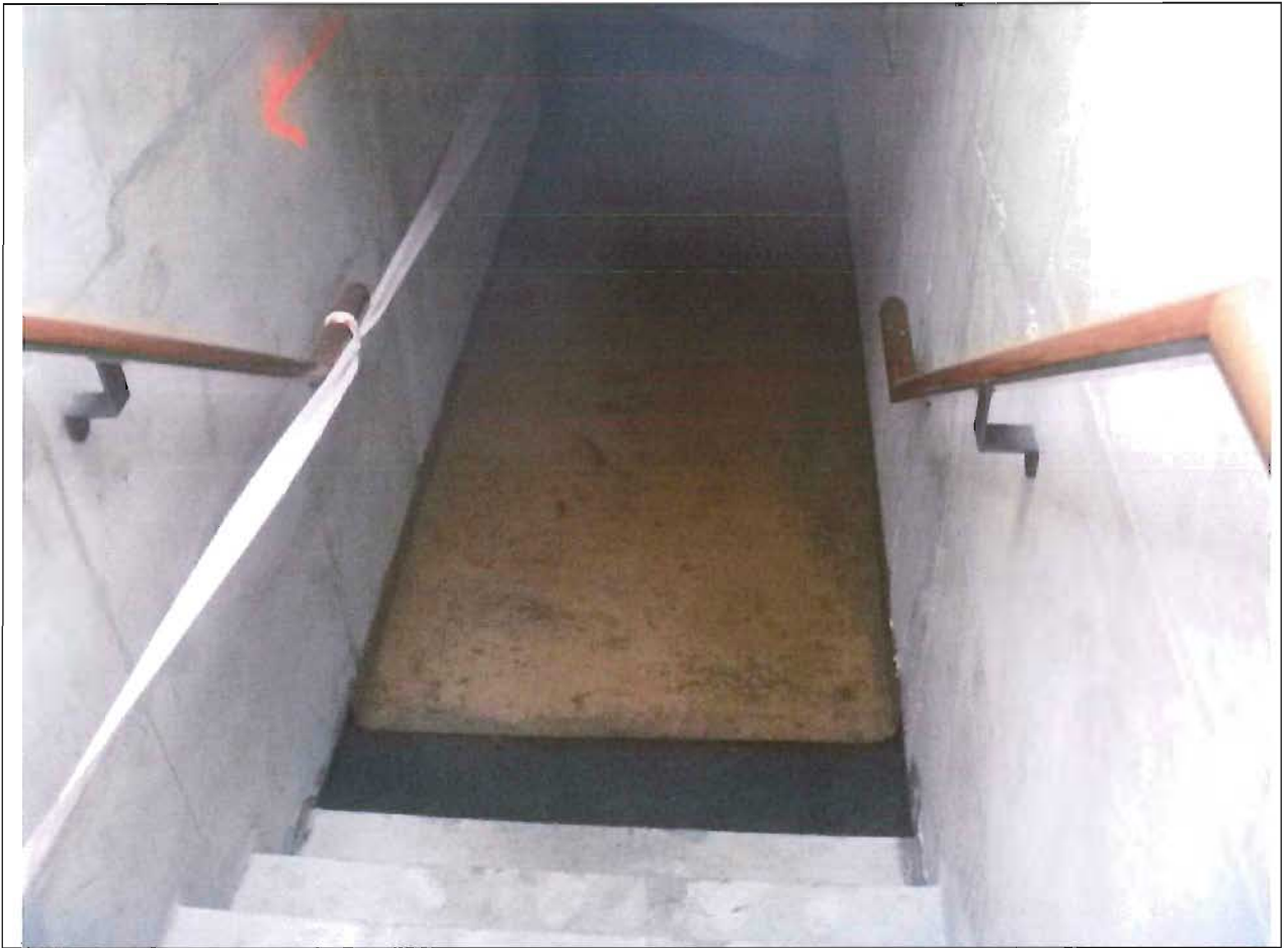
Photograph B - Approximately 100mm depth of water in tunnel
