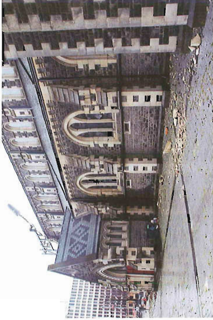
Figure 5 Buckling of the leaded lights to the south aisle windows has occurred, together with loss of the protective glazing, although these windows are capable of repair. Clerestory light above appear to be intact and to have suffered little or no damage.
