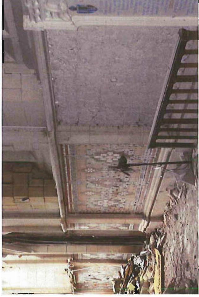
Figure 8 Damaged/fallen geometric mosaics to the south aisle.
