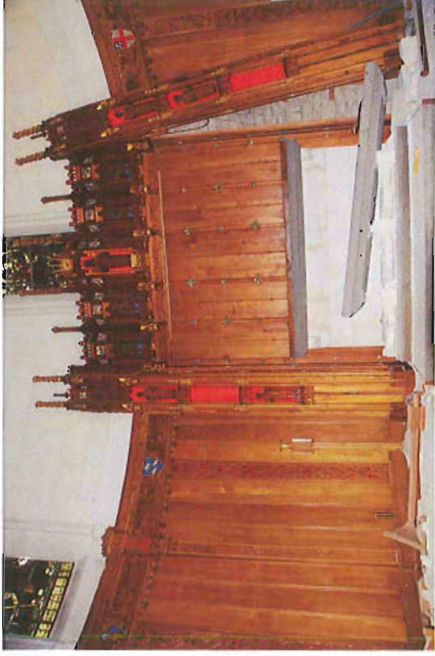
Figure 9 Collapse of the altar table
