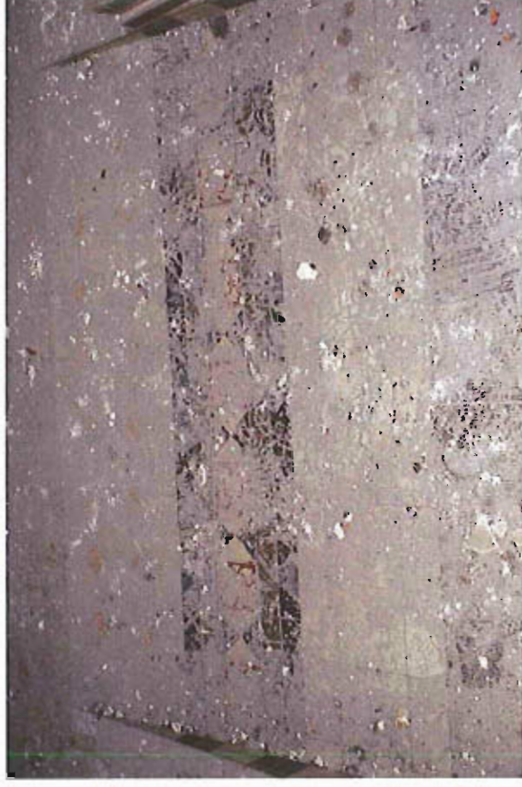
Figure 6 A section of the floor in the south aisle showing the extent of dust and potential for scraps/scuffing of the tiles even where masonry has not fallen
