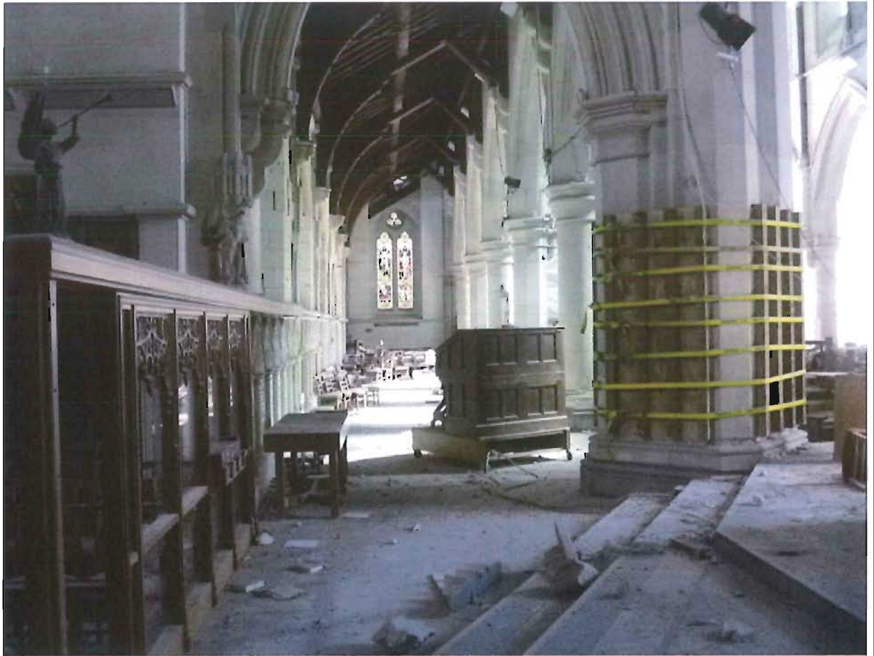
Photograph A – interior view of south exterior foundation and south row of column foundations
