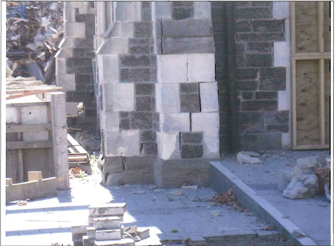
Photograph C – Shaking damage to the top of the foundation at the south west corner of the building
