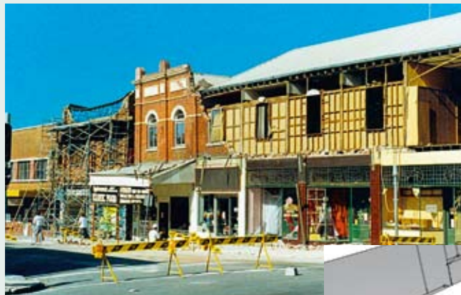
Union St shops damaged in the quake.
